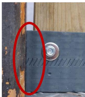
Too close to the hinge jamb on the pull side
