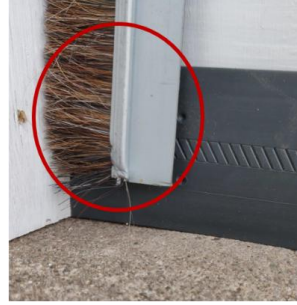
under brush side seal installed on the door
