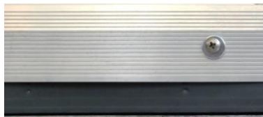
Damaged part of AIO hidden behind mounting strip
