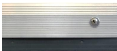
Damaged part of AIO hidden behind mounting strip
