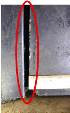
Side gap on the pull side
