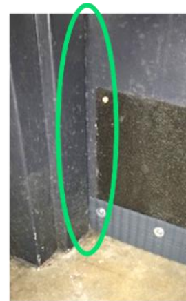
No side gap on the push side
