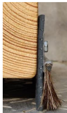
Same side installation
