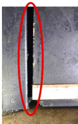
Side gap on the pull side
