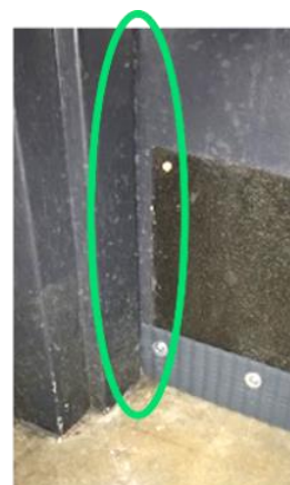
No side gap on the push side
