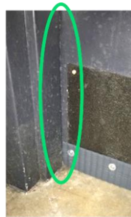
No side gap on the push side
